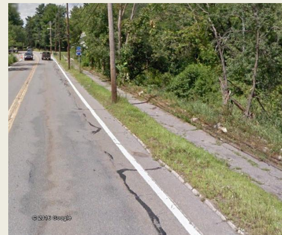
Sidewalk on north side of King St just west of Castle in the Trees Playground.
